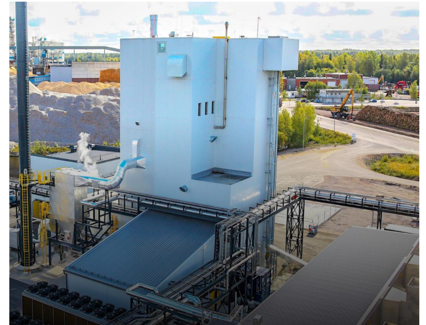
Existing pyrolysis plant in Gävle, Sweden, with capacity 40 000 tons of biomass per year. Source: https://www.btg-bioliquids.com/plant/pyrocell-gavle-sweden/
